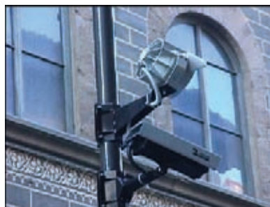
Typical ALPR camera and illumination device.
