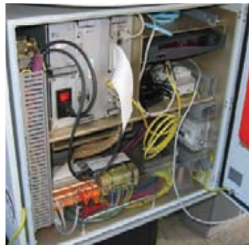
Centralized processing equipment.
